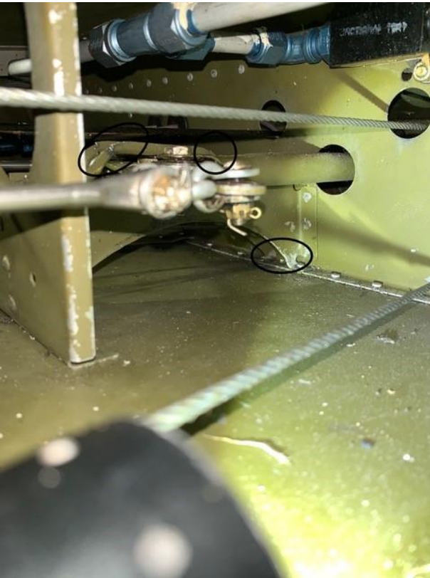
Photo 1 : Elevator Bellcrank and Bracket Assembly - Cracks found in upper bracket P/N 0411290 and lower bracket P/N 0411289-1.
