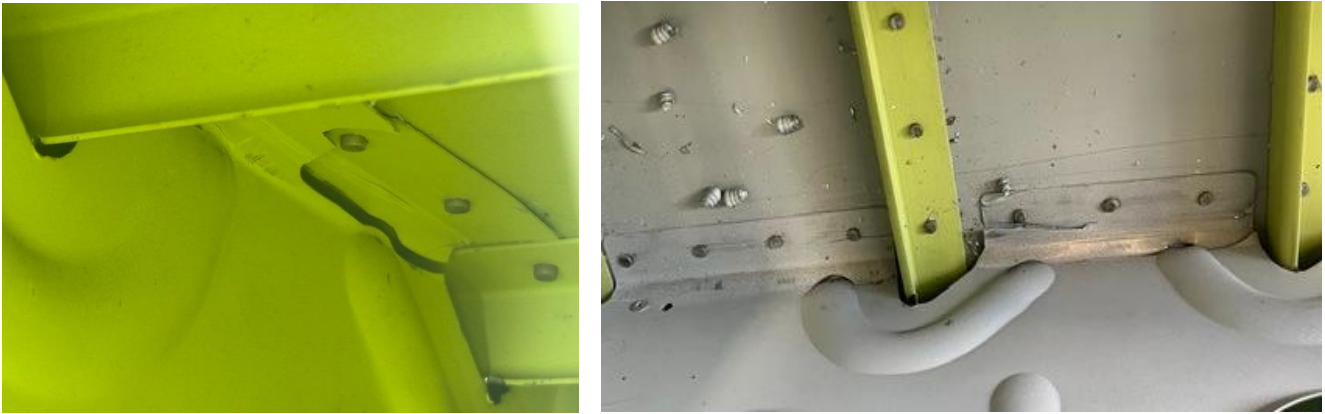
Figure 2 – Rib #2 LH and RH cracking 1 st aircraft.
