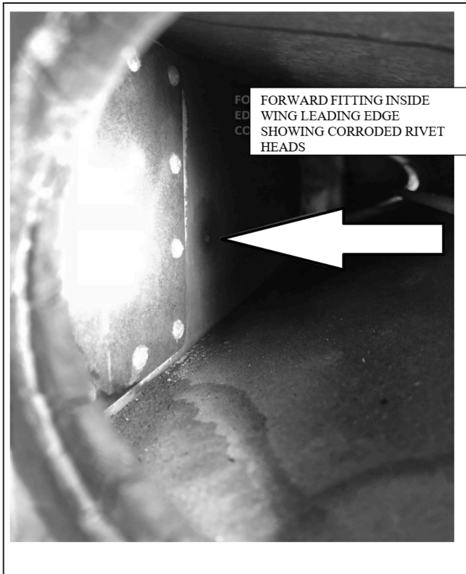
Figure 3. Wing Interior Showing Galvanic Corrosion
