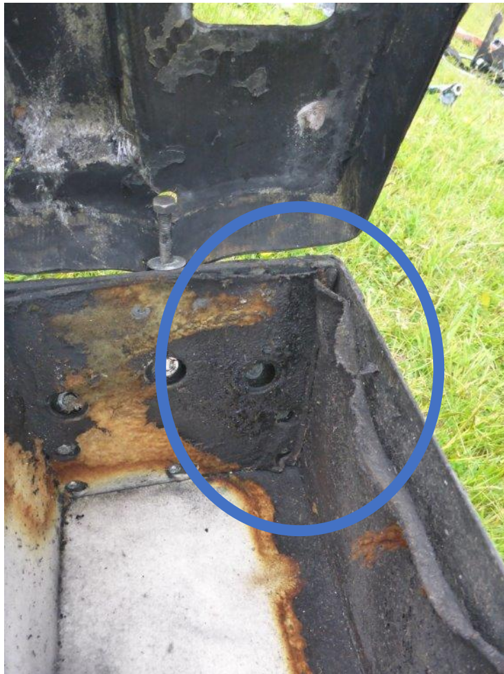
Figure 3: Origin point of the battery fire
