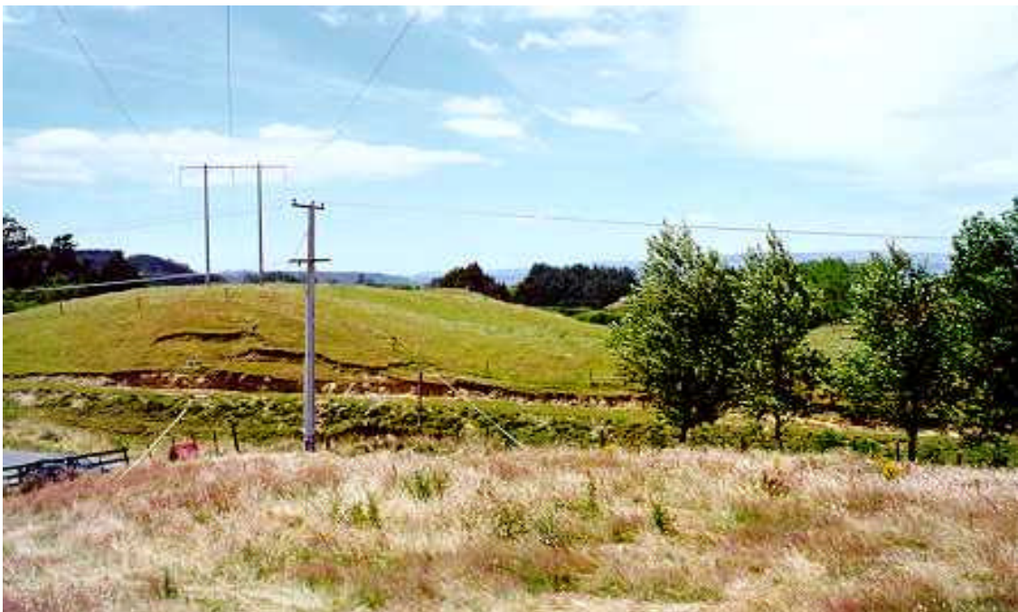
View to the south-east, looking across Jackson Road, showing the relationship between the 11 kV (bottom) and 110 kV (top) lines after the 11 kV pole had been replaced. The helicopter approached left to right, striking the left-hand 110 kV conductor.
